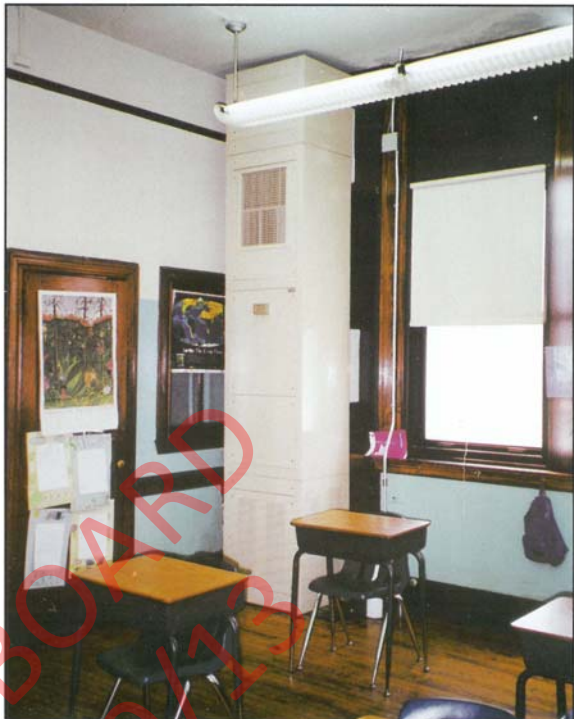
Interior view of a vintage school with vertical unit ventilators - free blown.
